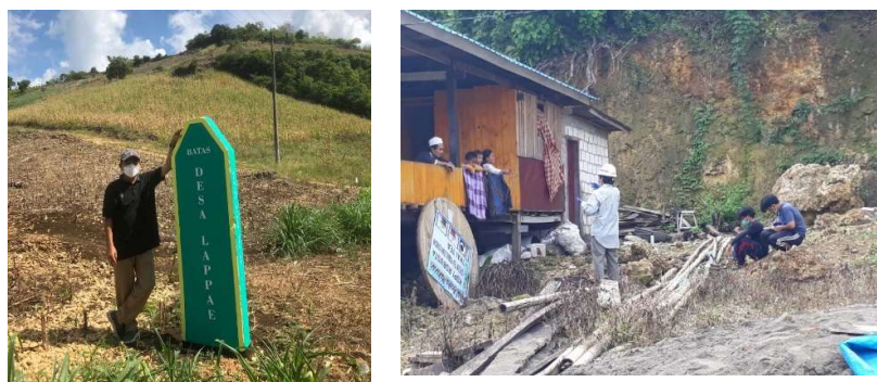
Figure 3. (Left) Rice field in the location. The sign of Lappae is inclined to the right, presumably due to land subsidence. (Right) Local residents reported land subsidence occurring behind their houses. The sign of land subsidence looked is visible in the cliff.
