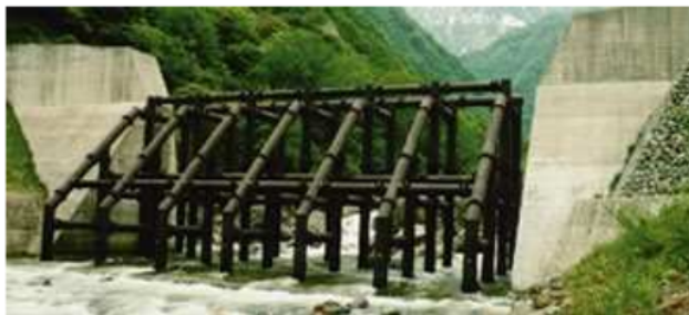
Gambar 4. Cek dam tipe grid pada Sungai Ikazawa Propinsi Niigata Japan (Source: Sustainability Report-Kobe Steel Group Sites, 2011)
