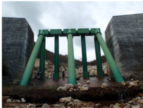
Gambar 5. Cek dam pipa baja di Sungai Hachimandani
